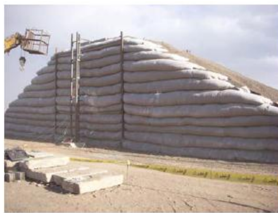
Fig.1. The general view of the prototype.
