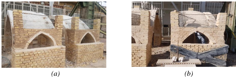
Figure 3. The stages of construction structure: a) Structure view of arch and rib cover; b) Structural view after reinforcement.
